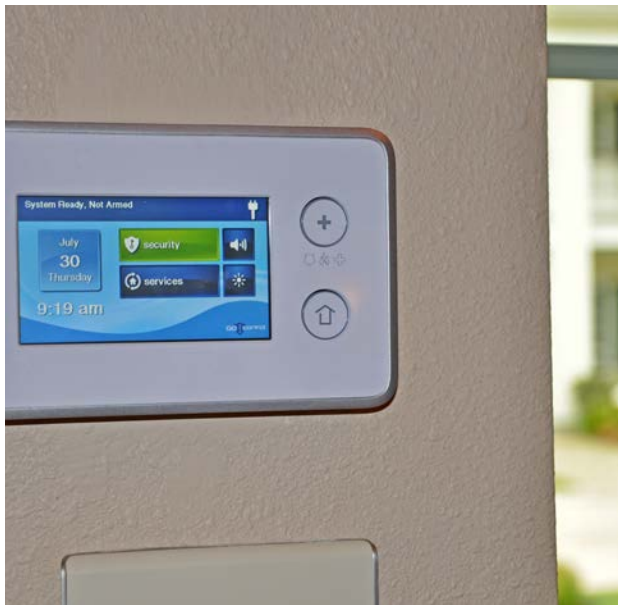
NRG empowers homeowners with energy management tools such as smart thermostats.
