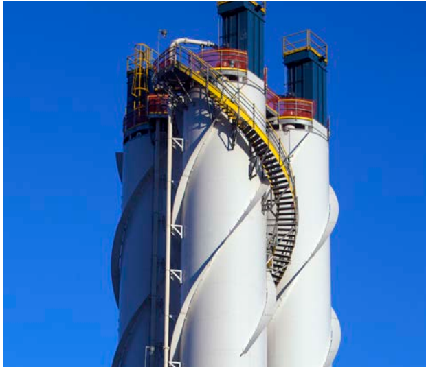
Installing BECs at our Waukegan Generating Station contributes to the overall modernization of our Illinois fleet.
