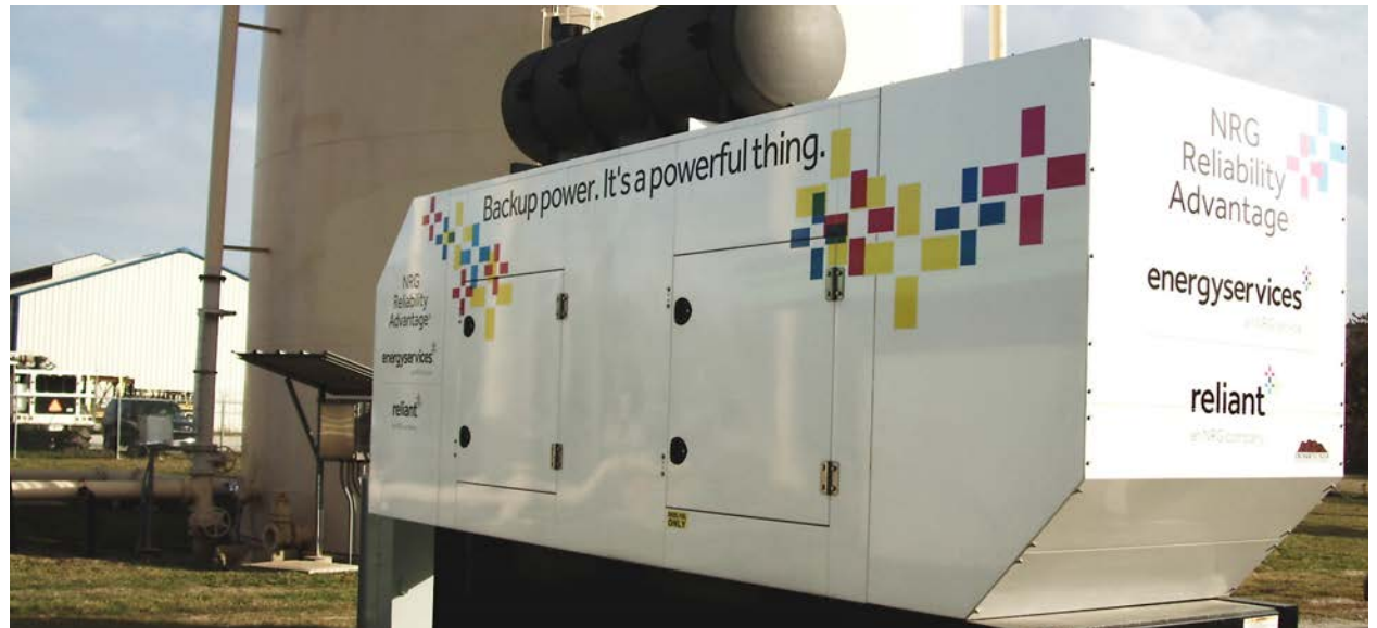
An NRG Reliability Solutions backup generator
