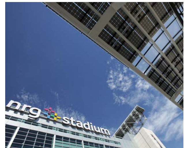
Our energy-efficiency project at Houston's NRG Park included installing solar panels atop one of the stadium entrances.
